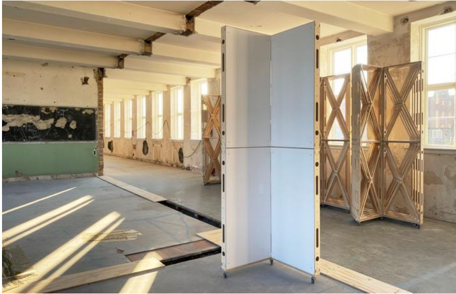
Figure 15. Development of the modules after prototyping phase (Danish cMDF – UC3)
